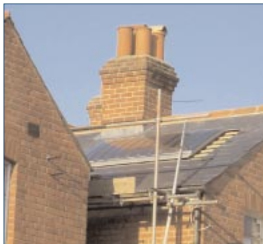
SHINE Project (Solar Housing through Innovation for Natural Environment) refurbishes forty-five Victorian terraced houses in Reading with energy efficient and renewable energy technologies. Here, a solar panel is installed in the roof of a house. Average annual heating and hot water bills are expected to be substantially reduced. The project is partly funded by the EU Thermie programme and similar activities are replicated in five other towns in Europe.
