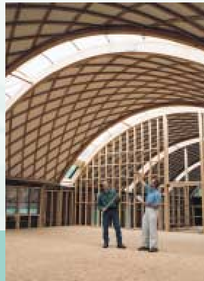
Woodland Enterprise Centre, Flimwell, East Sussex. SEEDA is co-funding this site which offers space for office and education facilities for woodland related industries in the the South East region.
