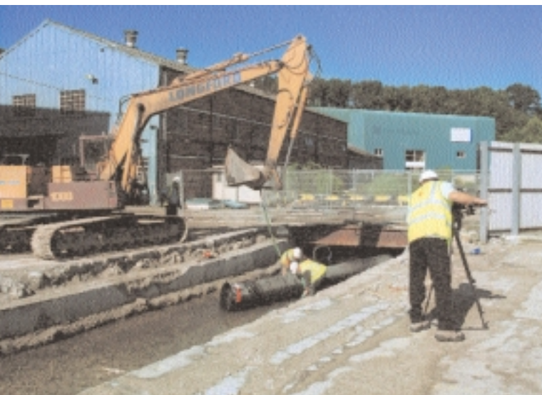
Concrete casing being removed to return the River Dour to its natural state.
