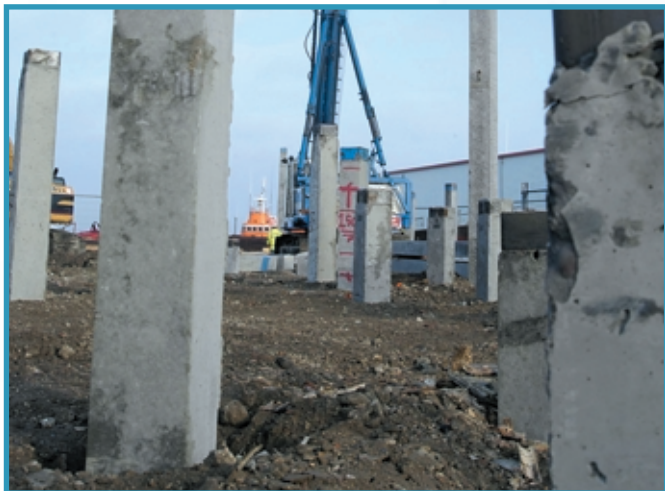
Pre-cast driven piles RNLI: Construction of lifeboat crew training college for the RNLI at Poole. Significant savings were made, both financial and environmental, by crushing concrete on site and changing pile design from CFA to driven pre-cast
