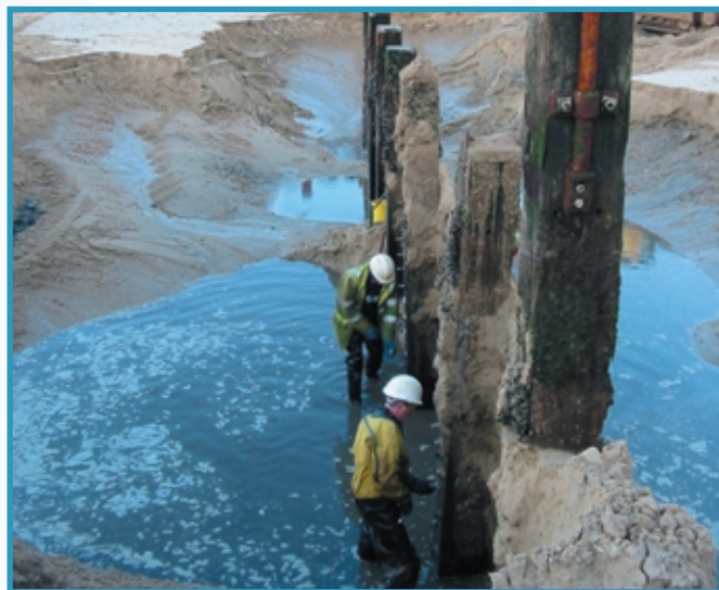
Timber for Recycling: Groyne renewal at Bournemouth for Bournemouth Borough Council. Timber is recycled for other uses
