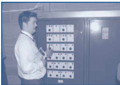
Thaddeus Dell, Crawley Borough Council, partner of the WSSBP, demonstrating the practical issues of energy saving during a SUMS site tour
